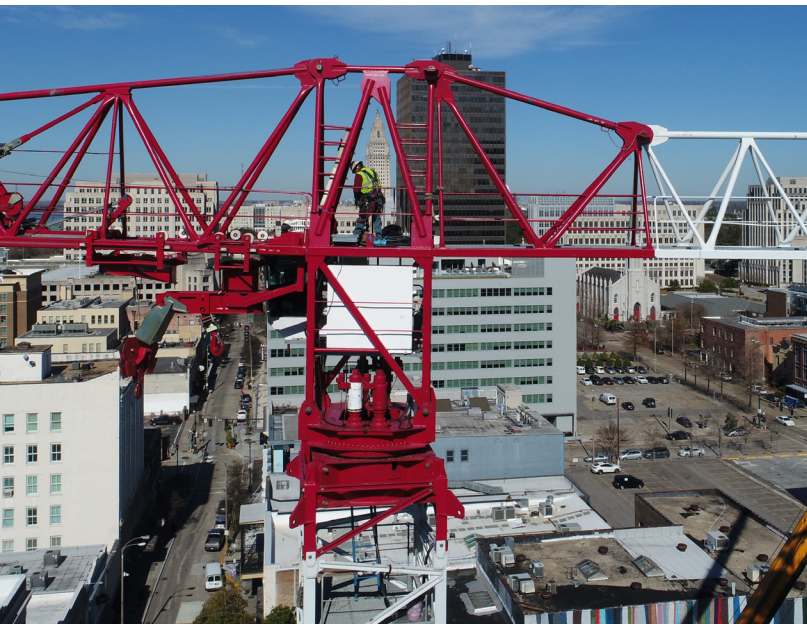
Above Left: Drones can be used to fly around construction equipment such as cranes and scaffolding. This saves safety professionals time and money. Photo courtesy of John Macahan/Ratcliff Construction.
